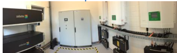
Speicher (Lilon 78 kWh)
